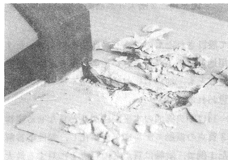
写真-23 階段近くの床の破損
